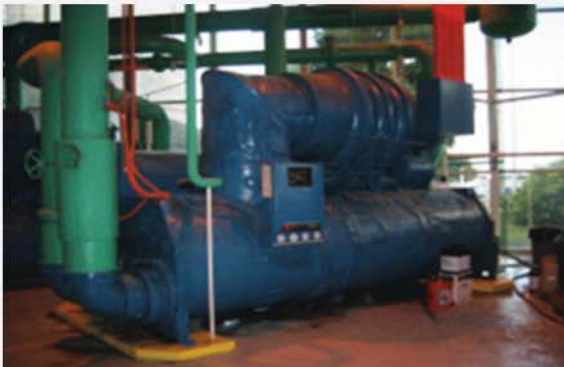
Figure 1 950-ton Trane Centravac Chiller
