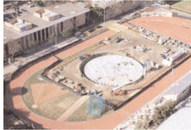
3.2 MG buried TES tank nearing completion beneath the track facility at the University of California in Pasadena, CA
